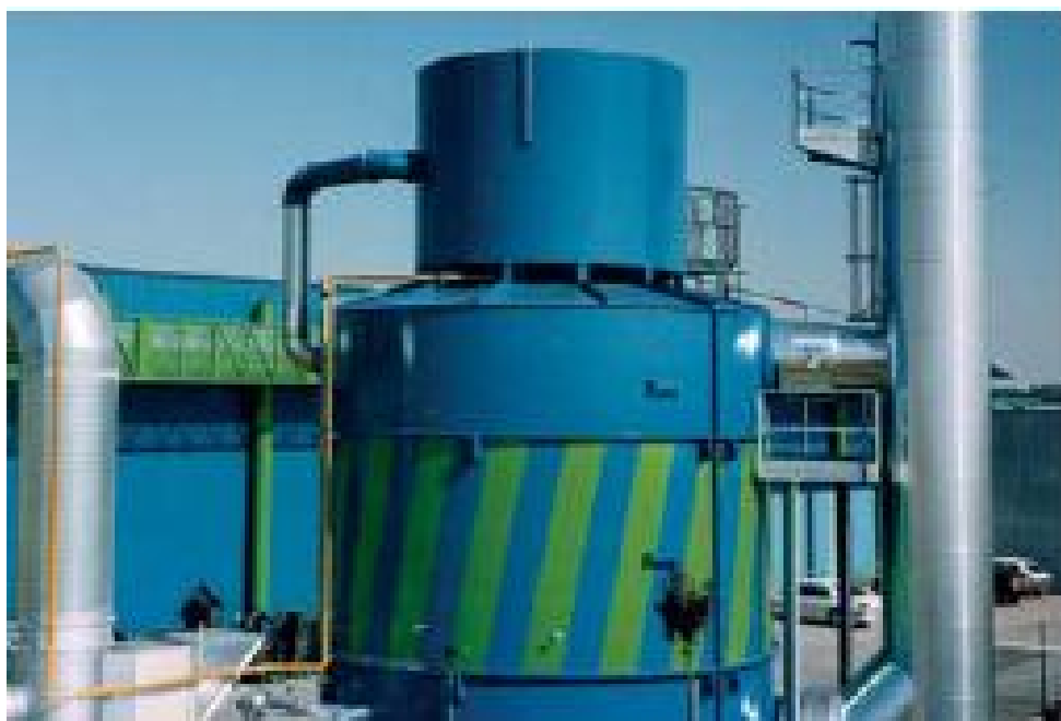
Рис. 2. VOC incinerator. Reducing pollution emissions from stationary sources.
